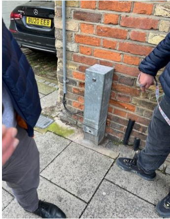
Example of feeder pillar on Ware High Street
