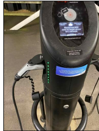
Example of a EV charging point
