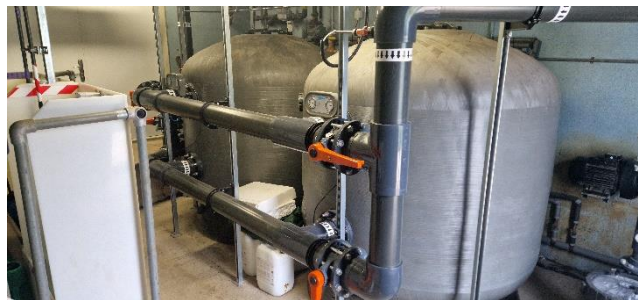
New Lido Filtration System
